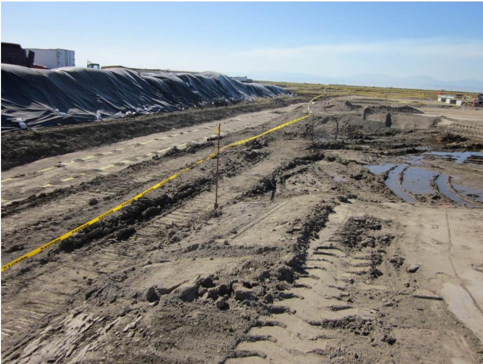
Photo 2: Backfilled portion of the trench at the south end of the Compressor Station site. Excavated soil has been covered to prevent displacement during rain events.
