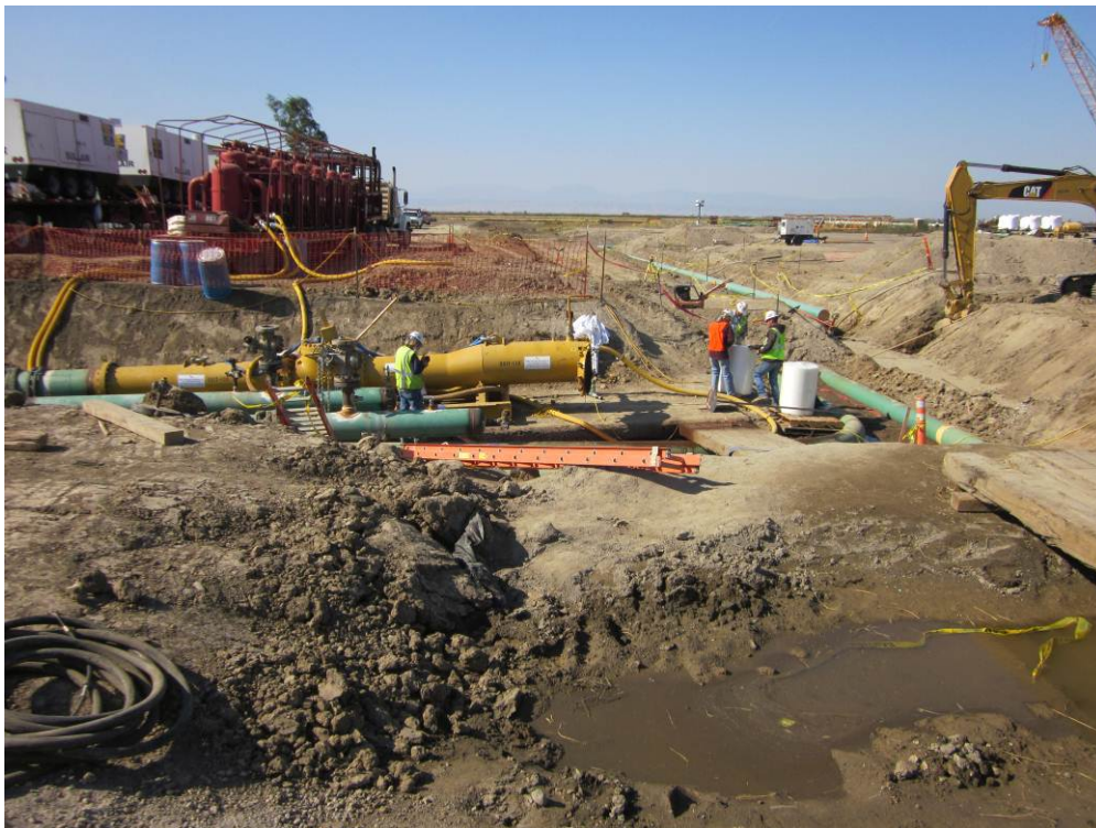
Photo 4: The terminus of the 24-inch natural gas pipeline at the Compressor Station. The pipeline is undergoing hydrostatic pressure testing.
