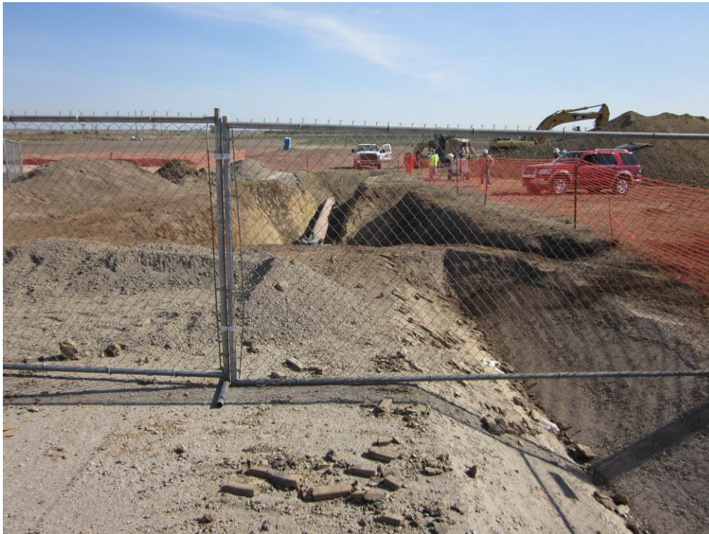
Photo 6: Natural gas pipeline terminus at the Metering Station. A small portion of the trench remained open for future tie-in at the Metering Station.
