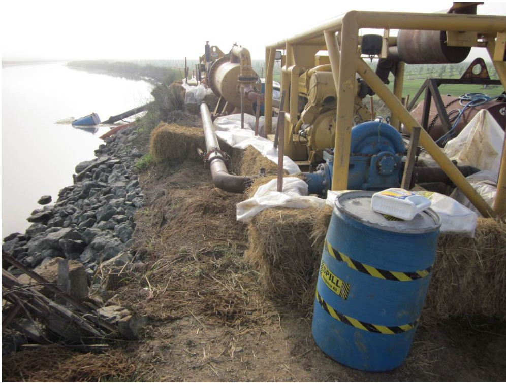
Photo 5: Pumps and compressors setup adjacent the Glenn Colusa Canal for hydrostatic testing of the pipeline. Secondary containment measures have been installed as required by Variance 14.
