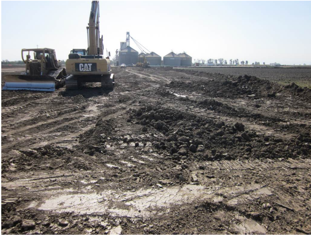
Photo 3: Pipeline right-of-way backfilling and grading between the Compressor Station and the Remote Well Pad site .
