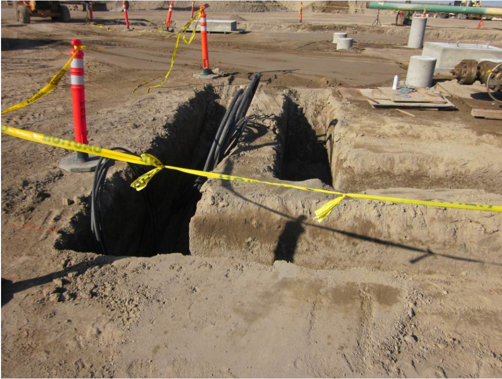
Photo 1: Trenching for buried electrical lines at the Remote Well Pad site. Trenches include wildlife escape ramps at trench ends.
